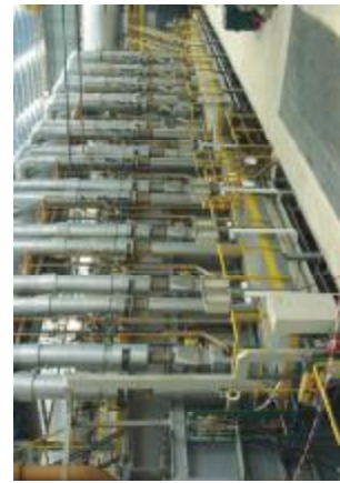
步进加热炉驱动 Step Heating Furnace Drive
